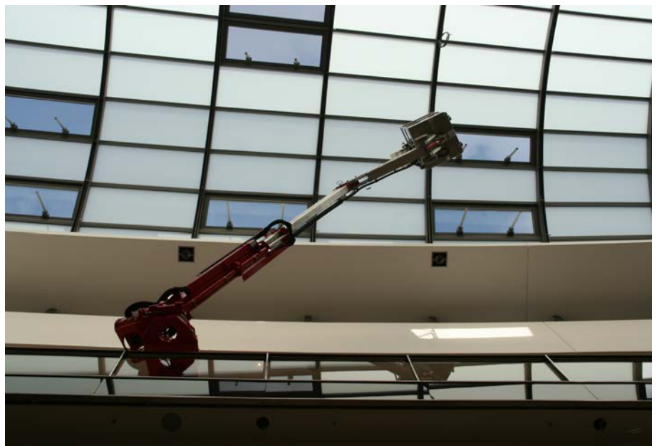
Working over railings
